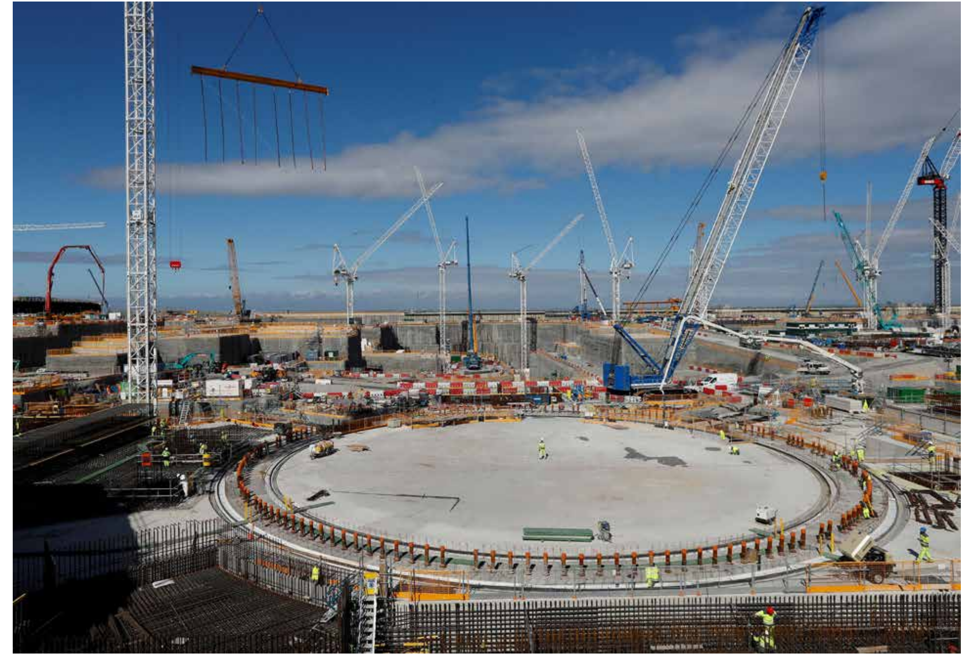
Workers at the nuclear reactor area under construction at Hinkley Point C nuclear power station site, near Bridgwater, south-west England, on 12 September 2019. The plant has been the most spectacular Chinese investment in Europe, with one-third of the project funded by China.
